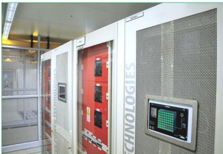
A UPS control panel.
